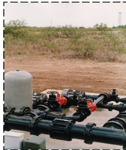
86 gallon tank replaces 30,000 gal standpipe
